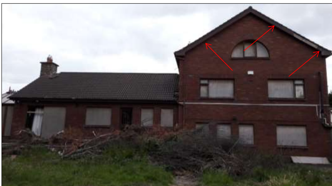
Plate 21. House 3 – rear view in 2018. Bats emerged from the fascia of the main gable as indicated by the red arrow).
