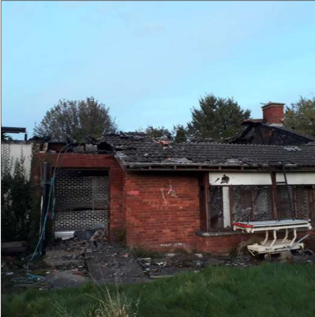
Plate 32. Rugby club building destroyed by arson - 2018.
